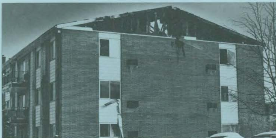
THE JANUARY FIRE destroyed Green Terrace Apartment Building 5, leaving several
