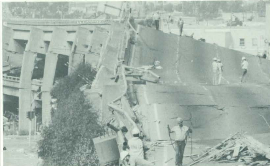
Rescuers searched for the hundreds of victims trapped under a one-mile section of Interstate 880 that collapsed during the Loma Prieta earthquake in San Francisco. —Associated Press
